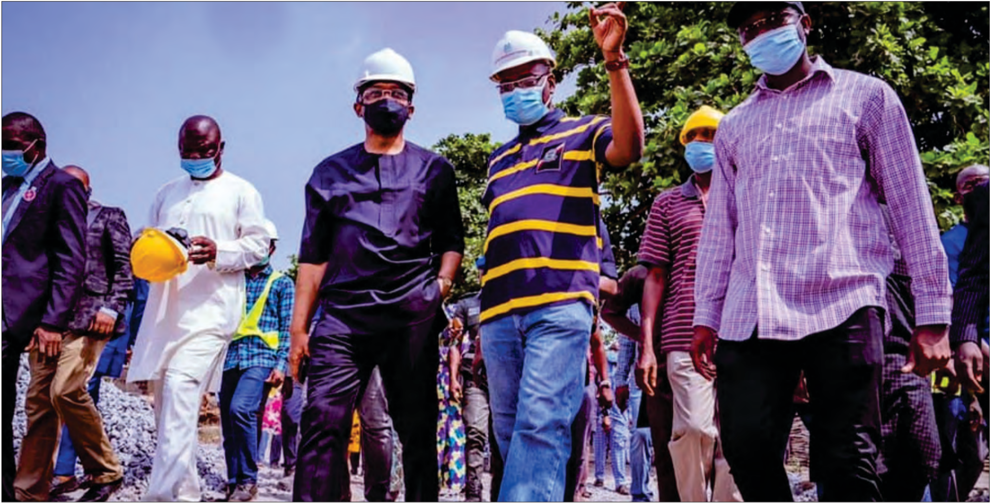
The visitation of the reconstruction and expansion work of Babs Animashaun road and bridge, and rehabilitation of network of seven roads at Ward F1, Surulere, comprising Nathan, Atan, Martins and Elizabeth Roads and others around Ojuelegba – Yaba axis.
